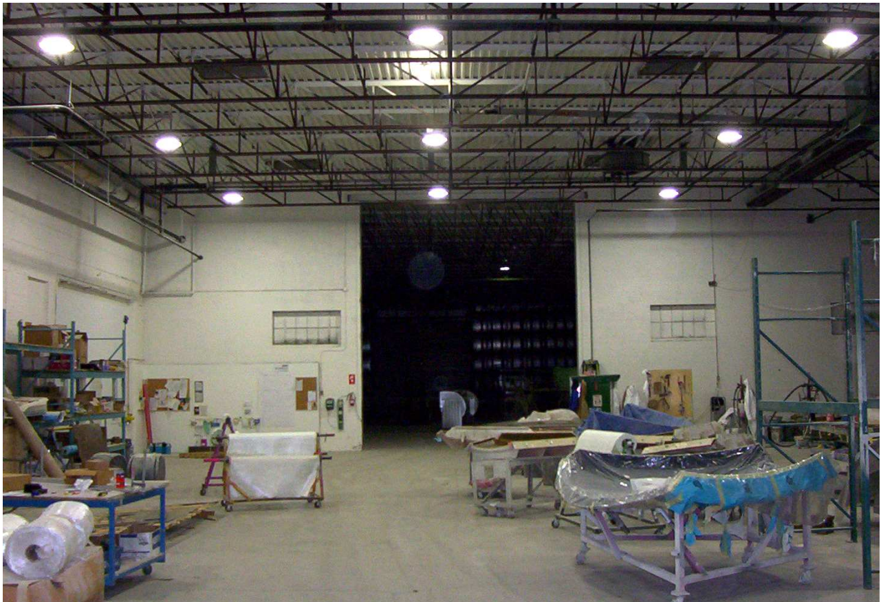
MAGNETIC INDUCTION LIGHTING HIGH-BAY LIGHTS IN OPERATION IN A MANUFACTURING FACILITY
